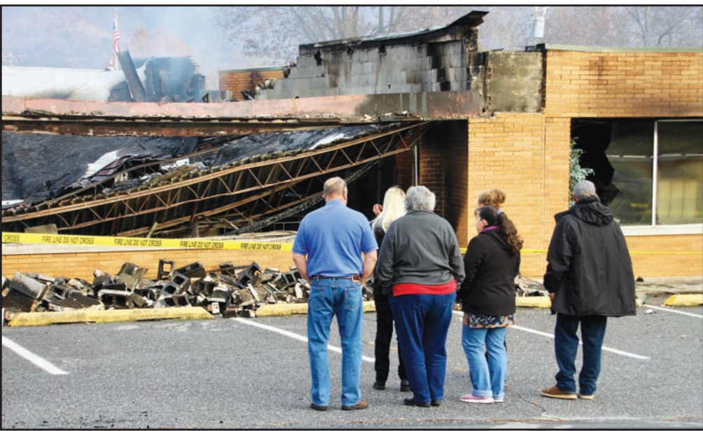
Spry Family Dry Cleaners owner and operator Mary Spry and supporters survey the damage at the family business the morning of the fire. Photo by Shawn Jarrard
